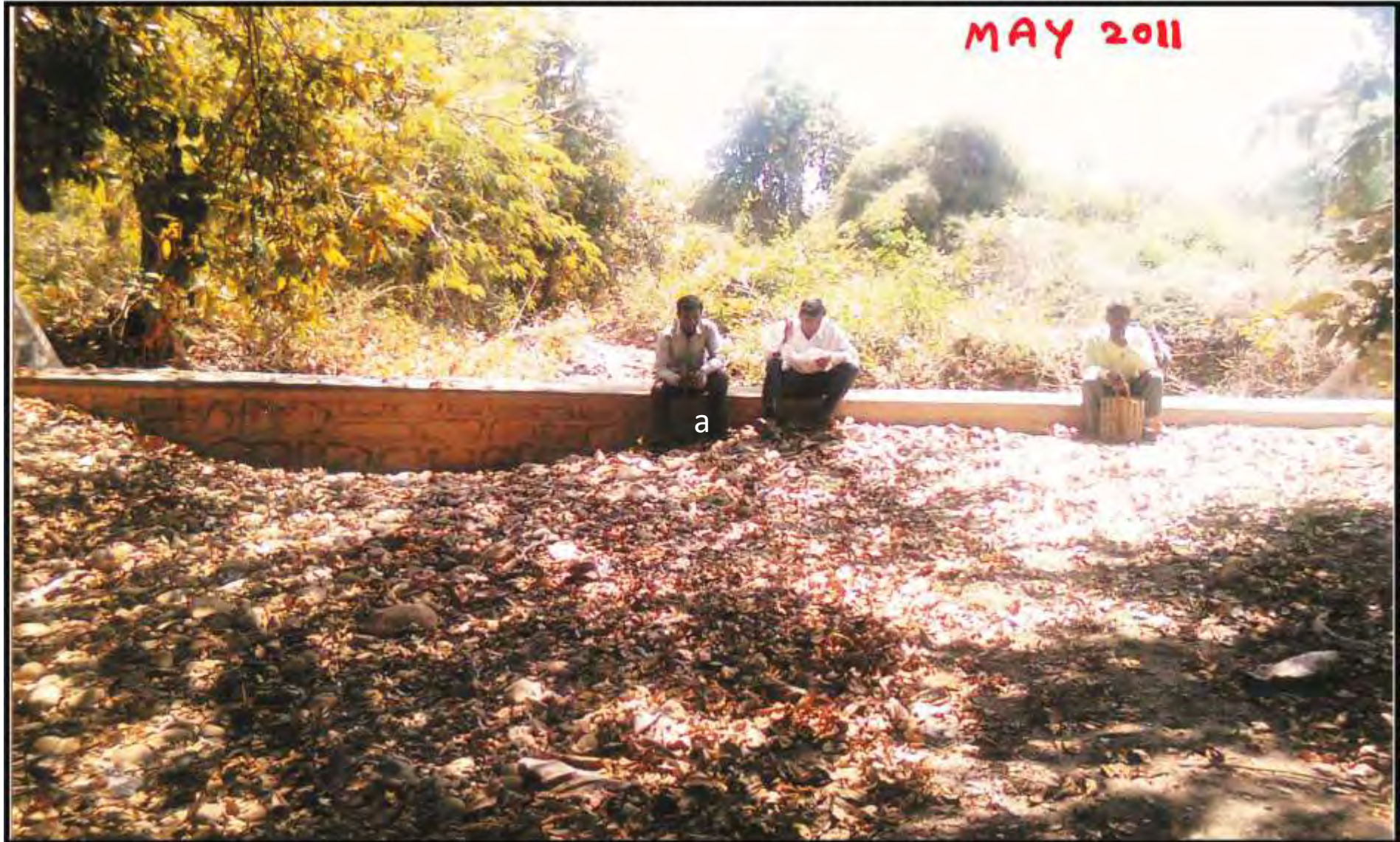
FULL DRY, SILTED BED, TAMASWADA NALA, TAH SELOO, DIST WARDHA USED TO BE IN MONTH OF OCTOBER BEFORE TREATMENT
