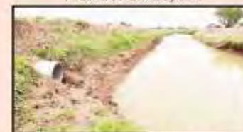
Rain Water Storage - 7 July 2017
