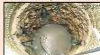
Recharge Well - Mahakal
