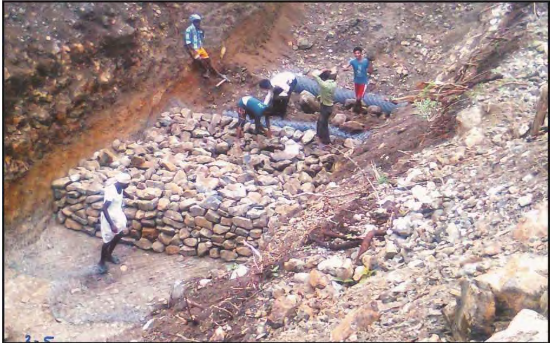
CONSTRUCTION OF GABIAN BANDH (TO STOP SILTING PROCESS TO REDUCE HIGH VELOCITY)
