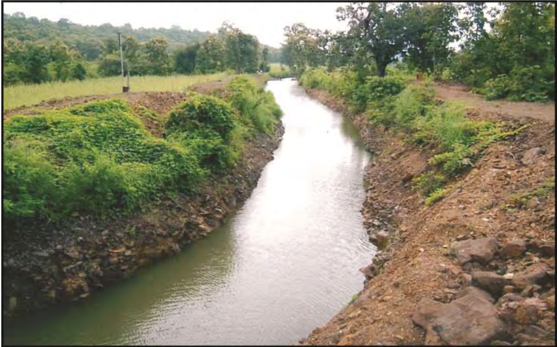
CREATED RAIN WATER STORAGE AT RIDGE PORTION
